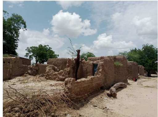
Damaged houses in northern Cameroon Source: Authors.
